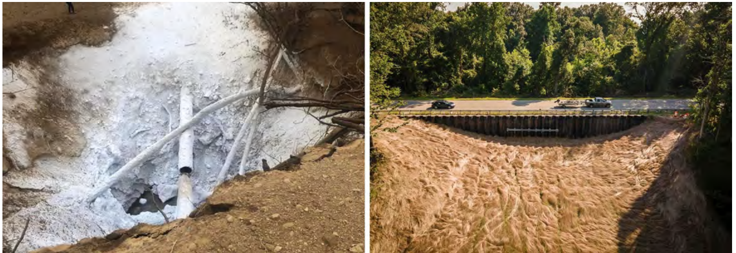
LEFT: The CO2 pipeline rupture. RIGHT: Vehicles pass over the pipeline explosion site in Satartia in July. Yazoo County Emergency Management Agency/Rory Doyle for HuffPost
